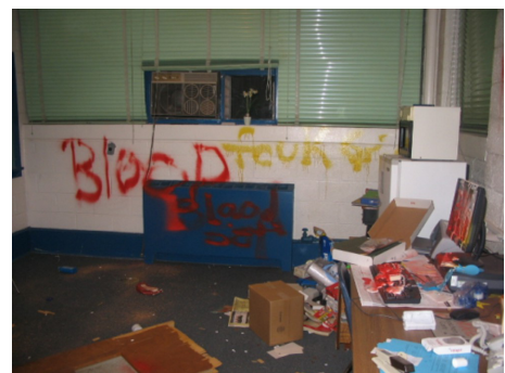
Gang Graffiti in a home in LaGrange.
