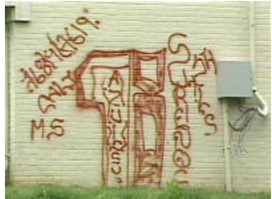
A graffiti reduction program is being developed.
