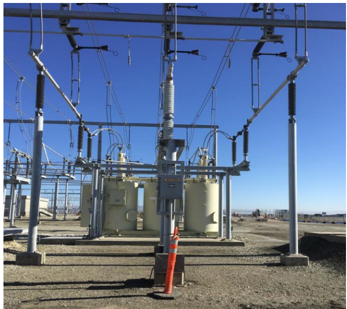
Figure 2: Circuit breakers (filled with oil)
