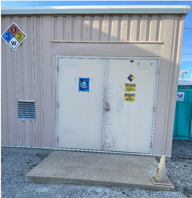
Figure 4: Battery room in Ravenswood Substation
