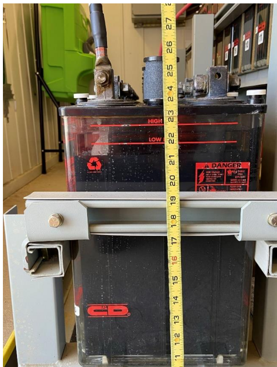
Figure 6. Batteries vulnerable to flooding levels of 2 feet
