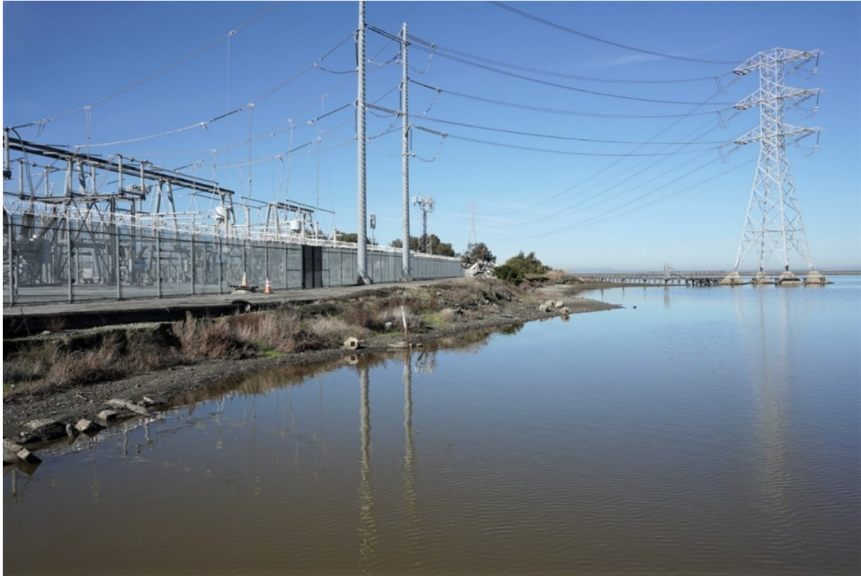
Figure 2b: Photos Taken at the Ravenswood Substation during High Tide on January 10, 2020
